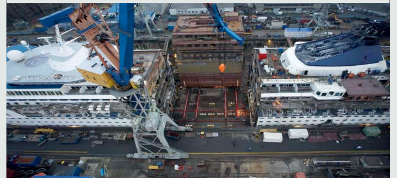
The new midship section of the «Norwegian Crown» is 30.2 m long, 28.21 m wide and without interior fittings weighs about 1,800 tonnes.
